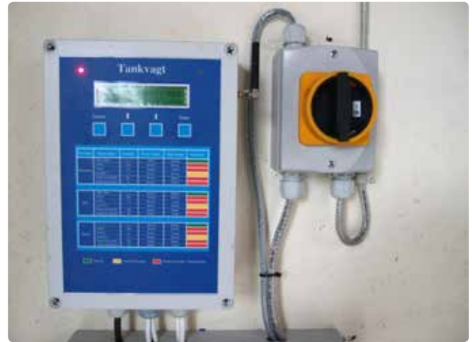
Fig 3. Example of approved tank guard.
