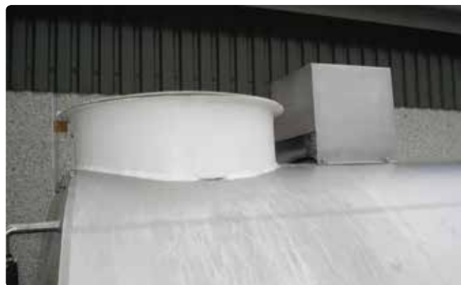
Fig. 7. Extra protection of a top mounted inspection hatch.
