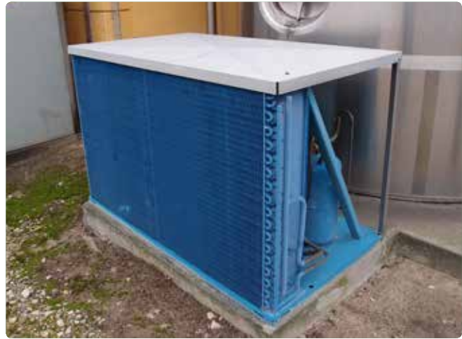
Fig. 12. Outdoor located cooling unit.
