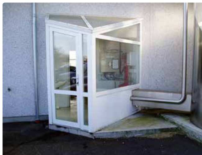
Fig. 10. Model 2. Free standing silo tank with outlet pipe and air vent led to the milk room.
