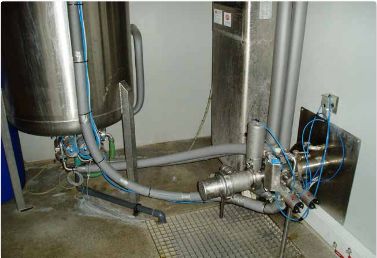
Buffer tank placed in the milk room. The tank is mounted on legs for direct emptying.
