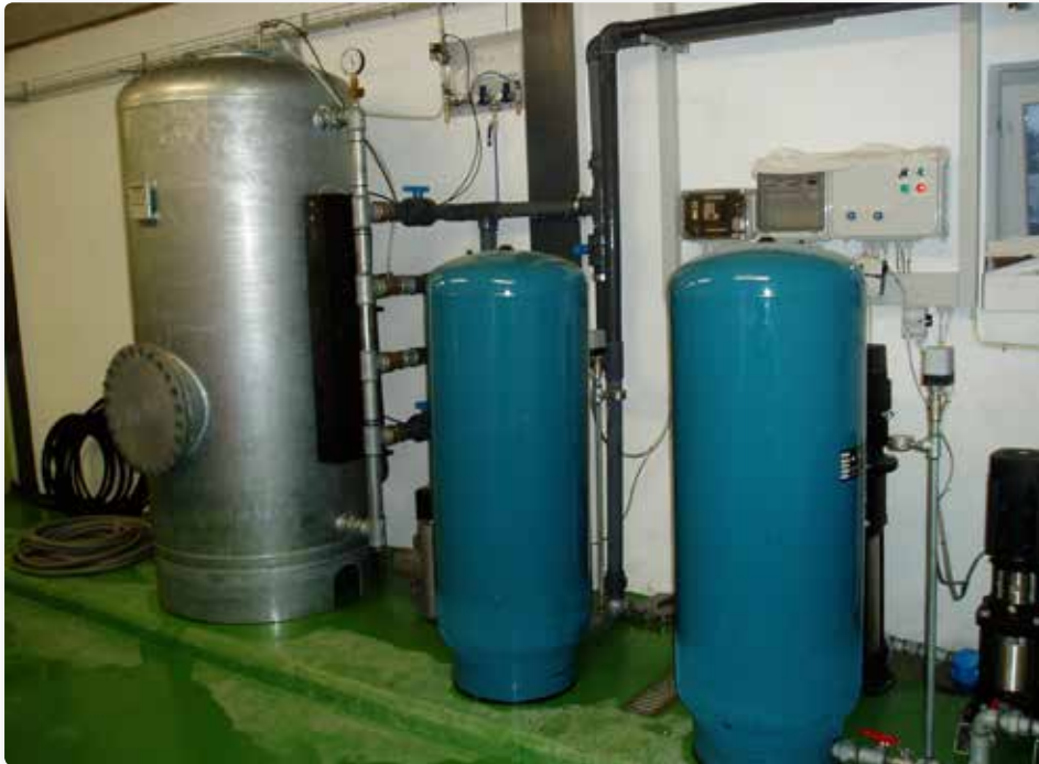
Plumbing with main inlet of water, water treatment and domestic waterworks.
