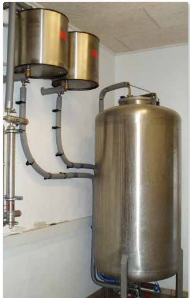
Tube coolers on AMS systems cooled with ice water.
