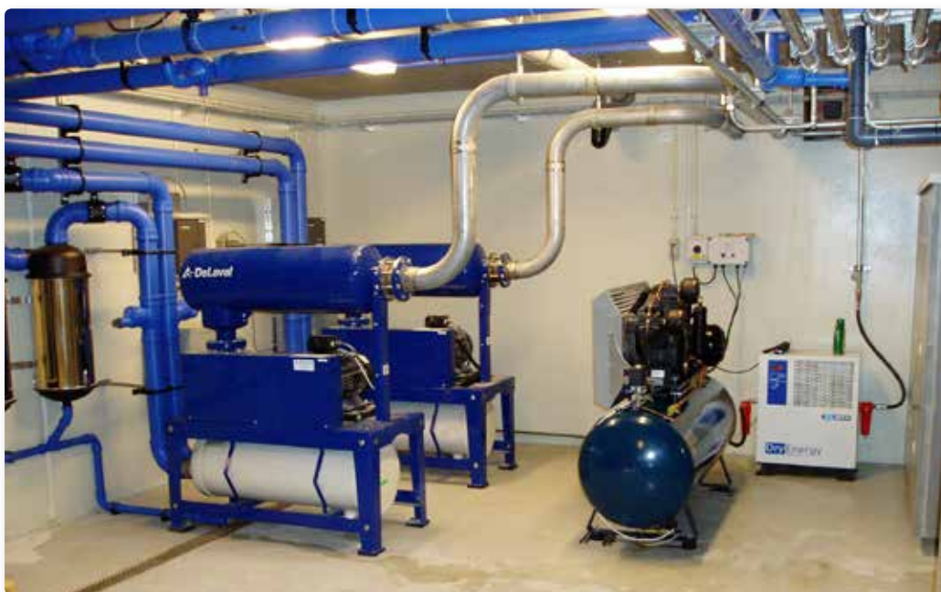
Equipment basement below milking centres with vacuum pumps and air compressor for the milking facility.
