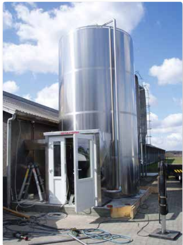
Silo tank with integrated collection room.
