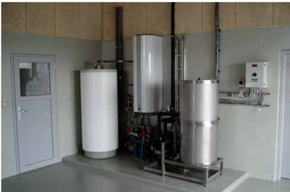
Plumbing in a cowshed with AMS Main water inlet, container for heat recovery, hot water tanks and ice water tanks. Unit for frost-proofing drinking-water in the cowshed.
