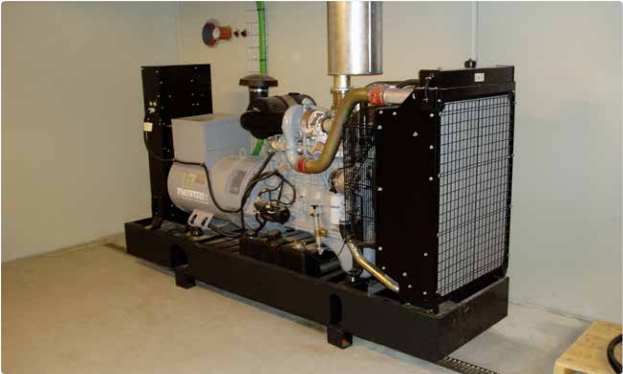
Emergency power generator with stationary diesel engine.
