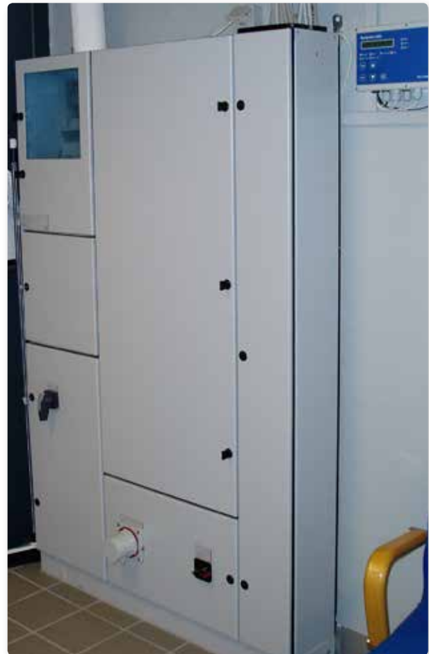
Electrical cabinet in office.
